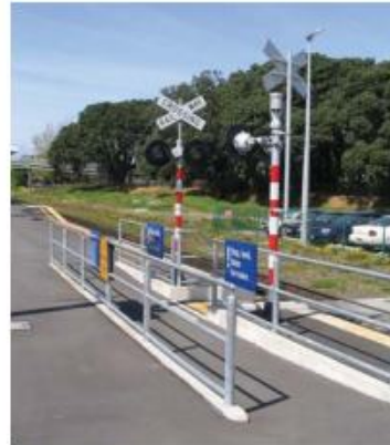
Photo 15.21 – Warning systems, Papakura (Photo: David Croft)
